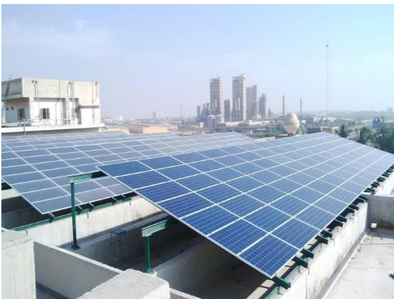
New solar capacities at our supplier's plant.
