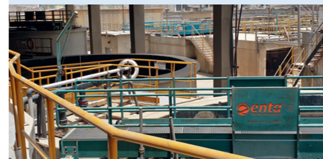
12 Dibella’s Pakistani towelling manufacturer has installed a modern water recovery system following the completion of the develoPPP project.
